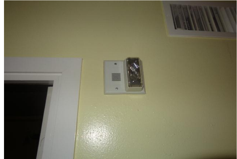
Photo #2 Smoke alarm strobe to be marked for removal by appropriate personnel.
