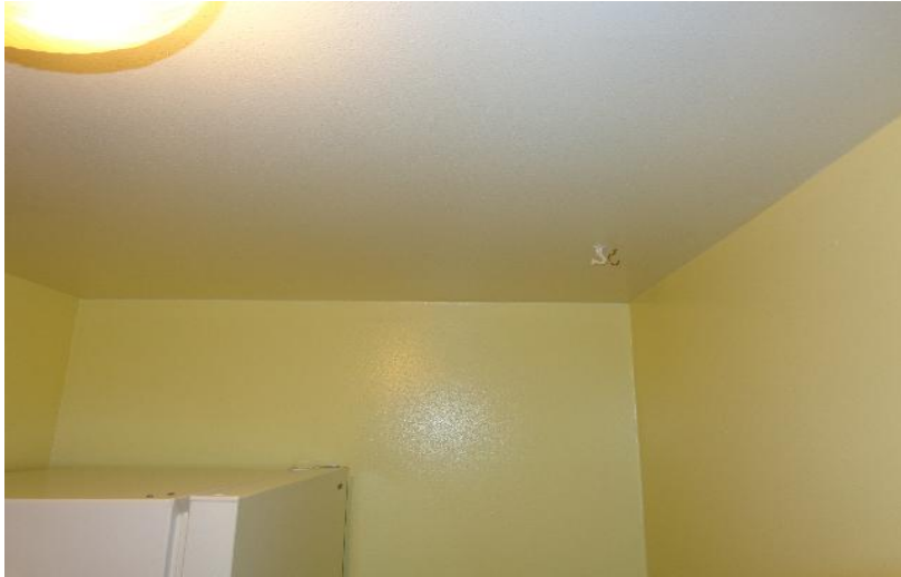
Photo #1 Drywall construction walls/ceiling to be marked for removal by appropriate personnel.
