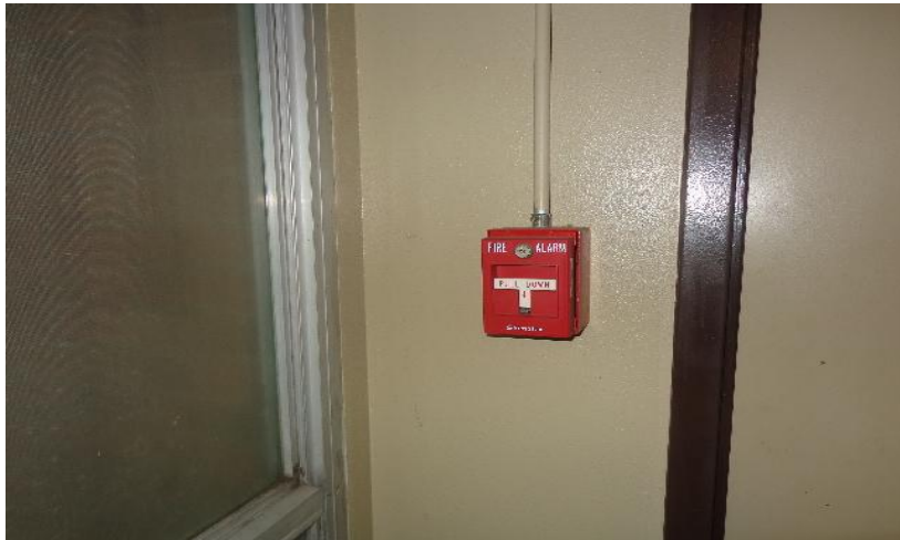
Photo #7 Fire alarm pull station to be marked for removal by appropriate personnel.
