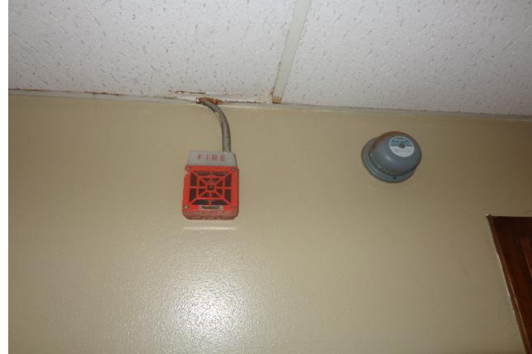
Photo #6 Fire alarm to be marked for removal by appropriate personnel
