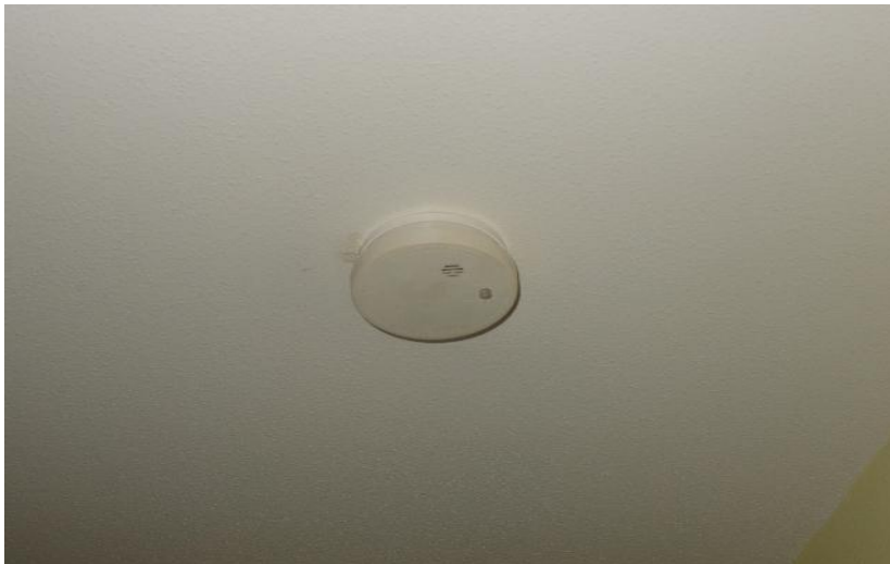
Photo #3 Smoke alarm to be marked for removal by appropriate personnel.
