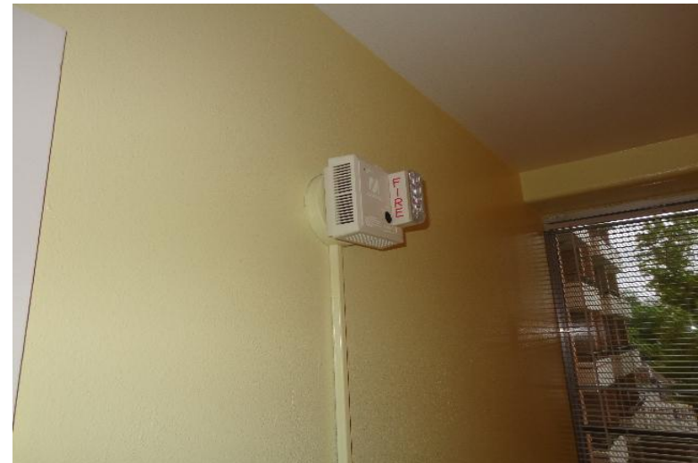
Photo #4 Smoke alarm strobe to be marked for removal by appropriate personnel.
