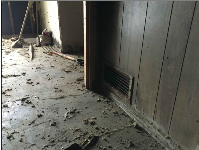
27: View of furnace grille vent.
