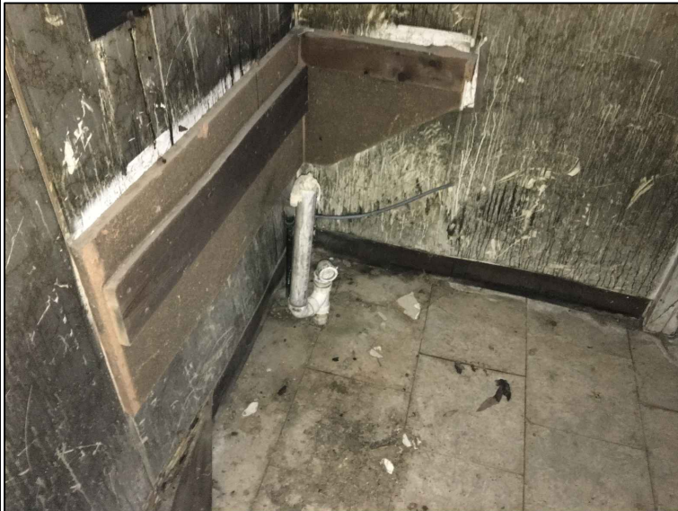
25: View of water piping associated with the women's bathroom.
