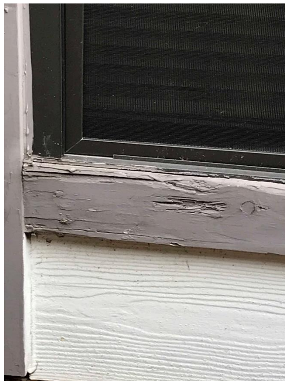
Typical wood to be repaired before paint
