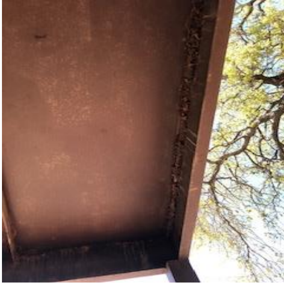
Typical rust under stair tower landing
