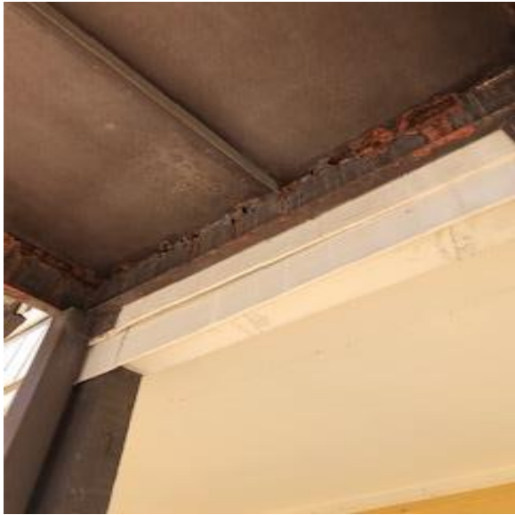
Typical rust under stair tower landing
