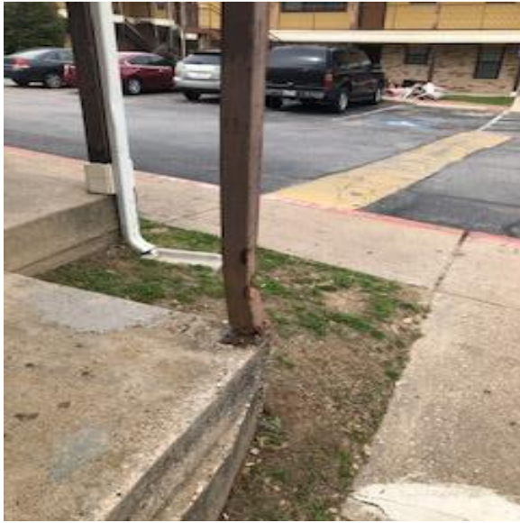
Stair column bent
