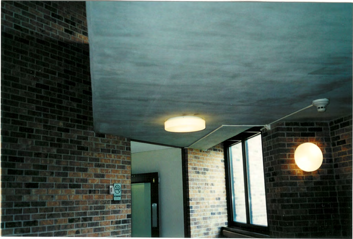
Plates 1 & 2: Showing asbestos containing ceiling texture material on the 3rd and 4th floor corridors respectively. (Typical).
