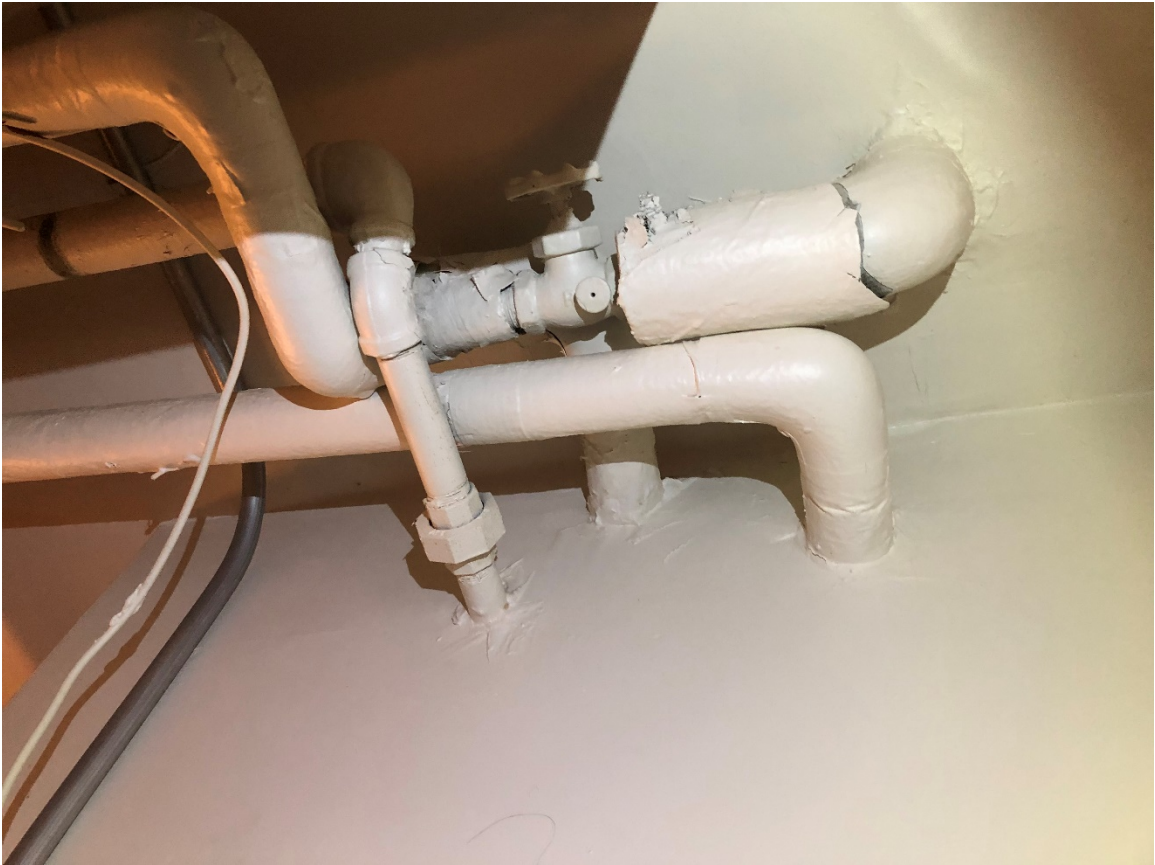
Photo 18: Pipe Fitting Insulation (Hard Elbow)
