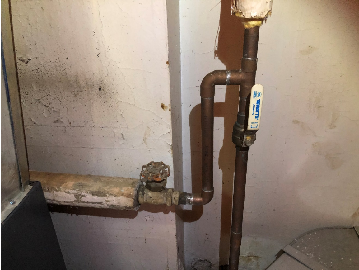
Photo 19: Paperwrap Pipe Insulation
