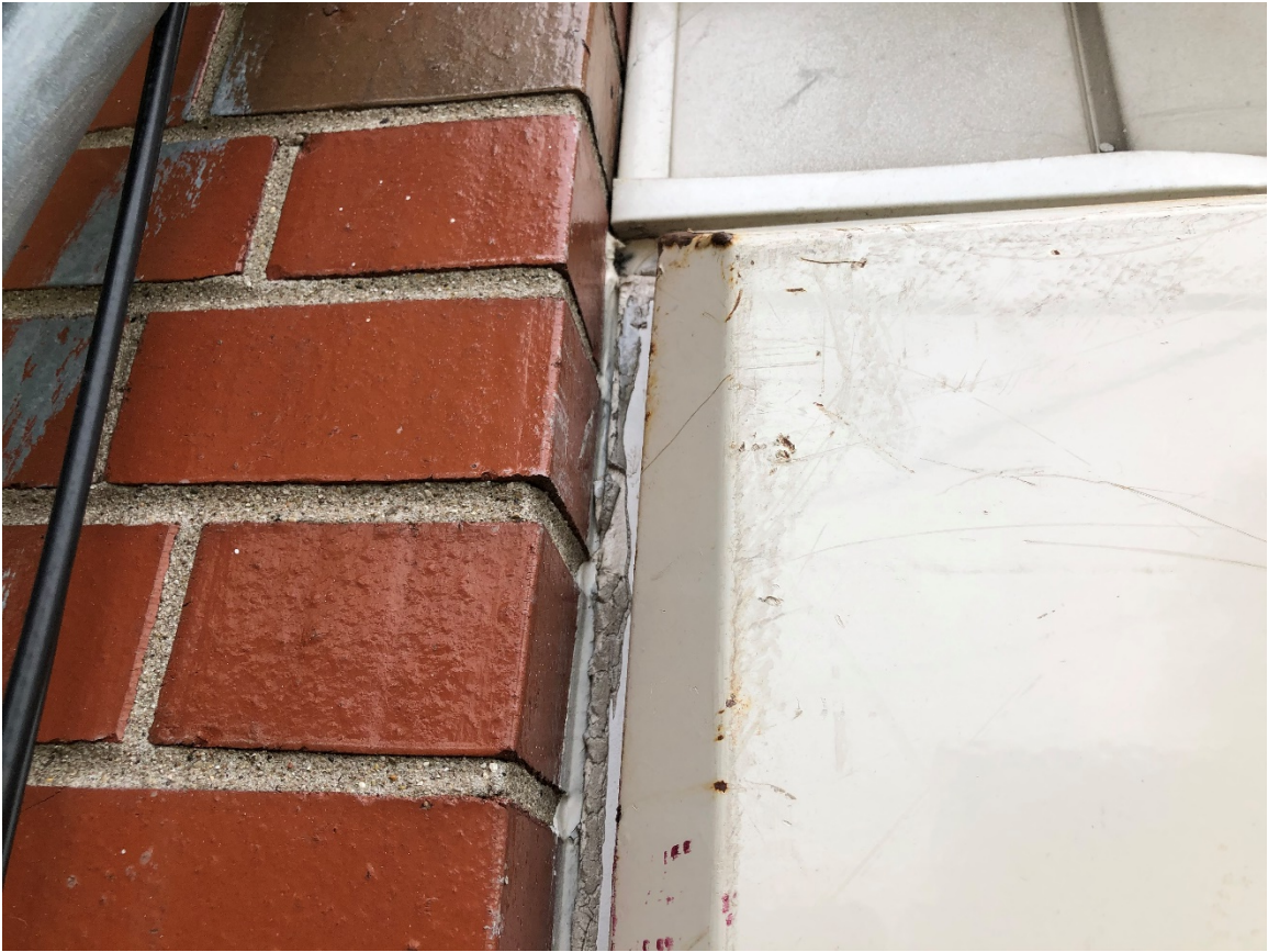
Photo 13: Exterior Siding Caulk
