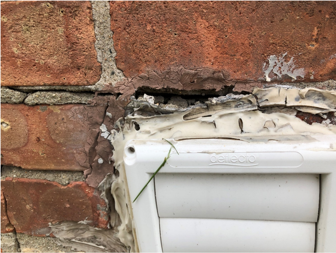
Photo 15: Exterior Vent Caulk
