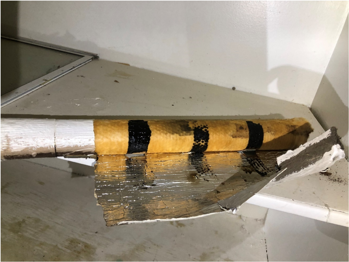
Photo 3: Black Tar on Fiberglass Insulation
