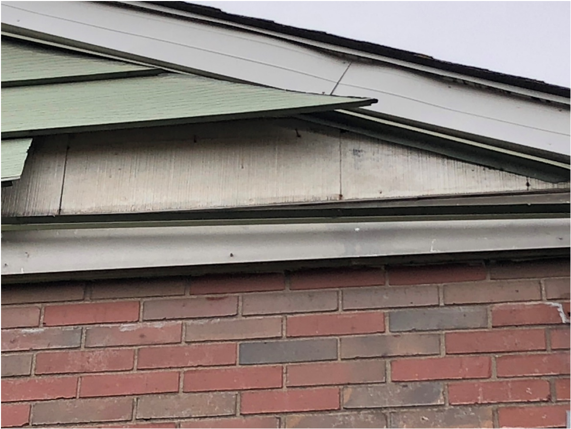
Photo 14: Exterior Transite (behind Vinyl Siding)
