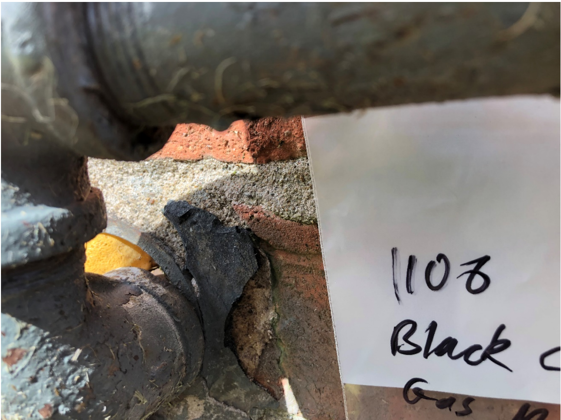
Photo 12: Exterior Black Gas Pipe Caulk
