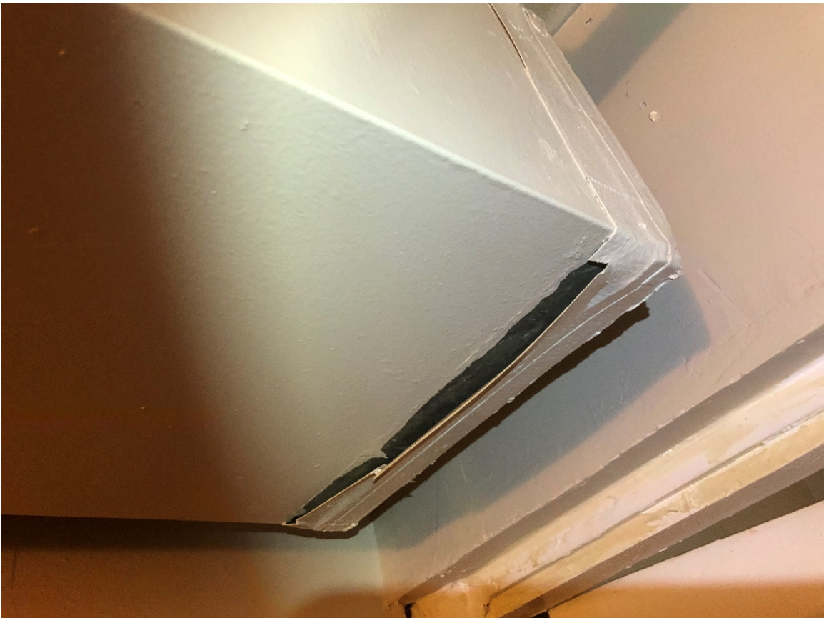
Photo 20: Paper Duct Wrap
