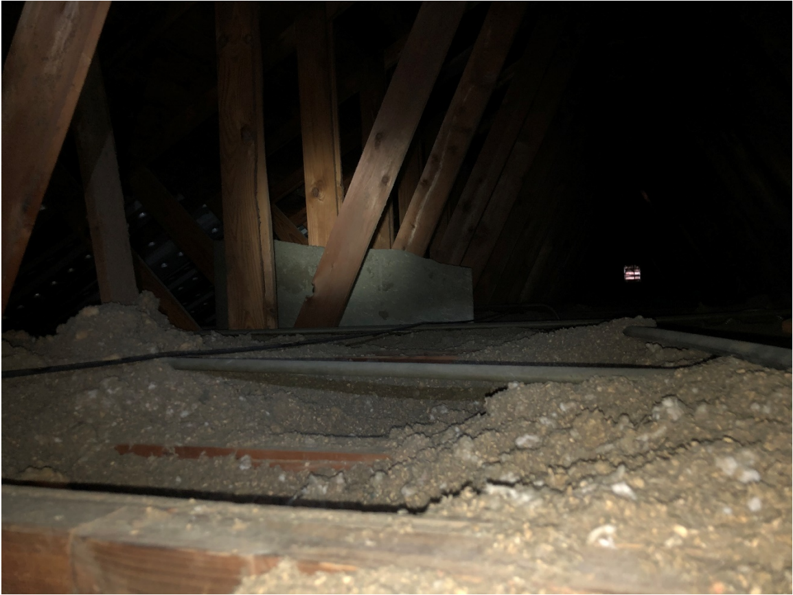
Photo 23: Transite in Attic
