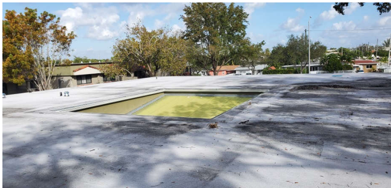
Photo 6: No asbestos identified in the samples collected of the roofing materials during this inspection.
