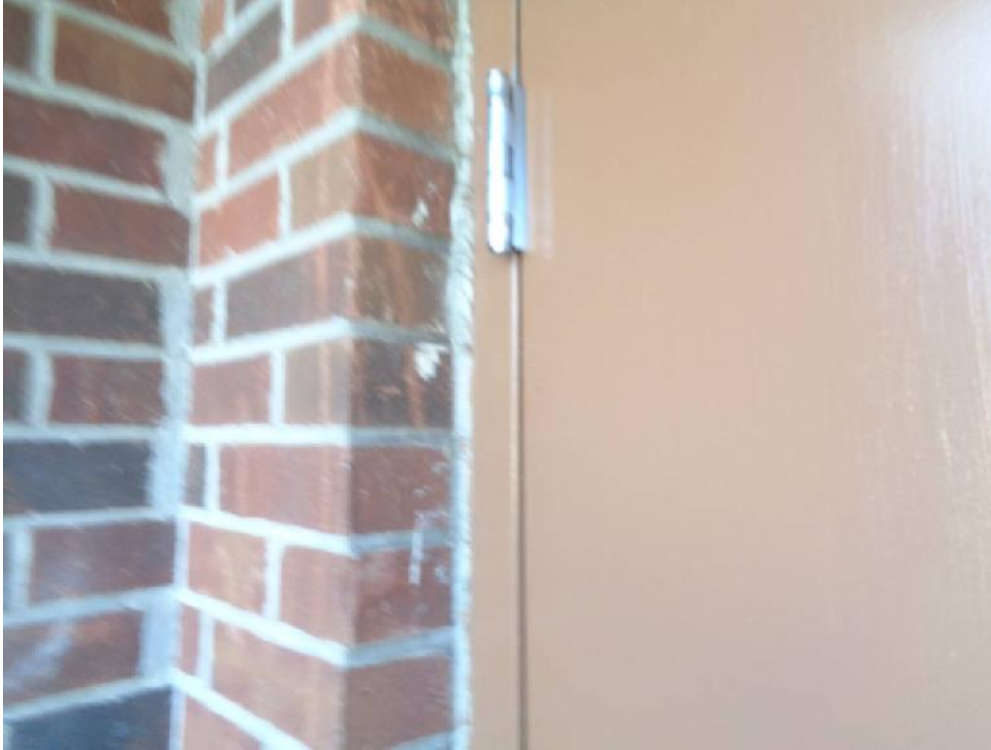
Photo 25: Typical view of white door caulk (DCA, non-asbestos) of the exterior doors.
