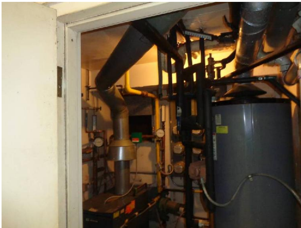
Photo 8: Typical view of common area boiler room showing drywall in the boiler room and hallway (DWA/DWB, non-asbestos).
