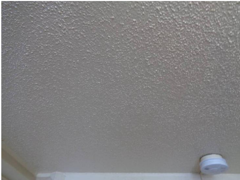
Photo 20: View white ceiling texture (CTA, asbestos containing) from the common areas of 9842 Oak Place Court.
