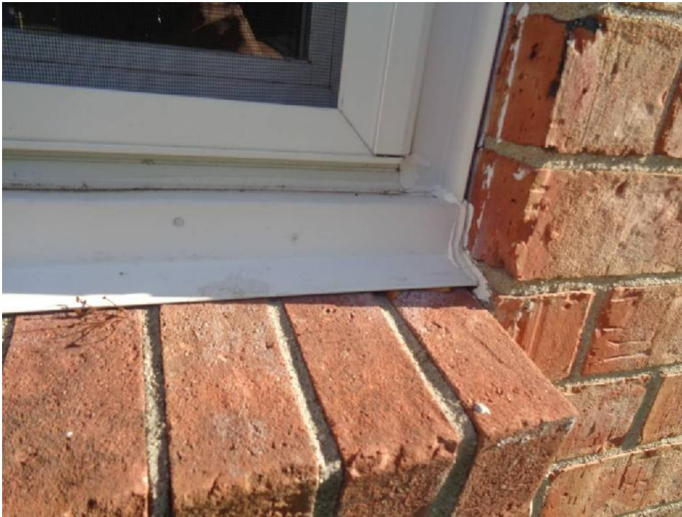
Photo 26: Typical view of white window caulk (WCA, non-asbestos) of the exterior windows.
