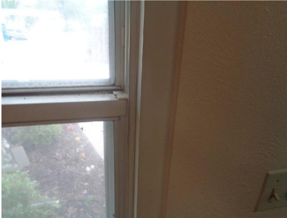
Photo 13: Typical view of interior white window caulk (WCA, non-asbestos) found throughout the facility.
