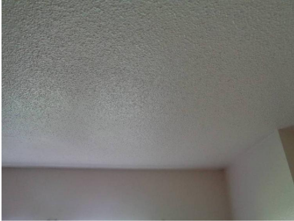
Photo 23: View of white ceiling texture (CTA, asbestos containing) from Unit C of 9842 Oak Place Court.
