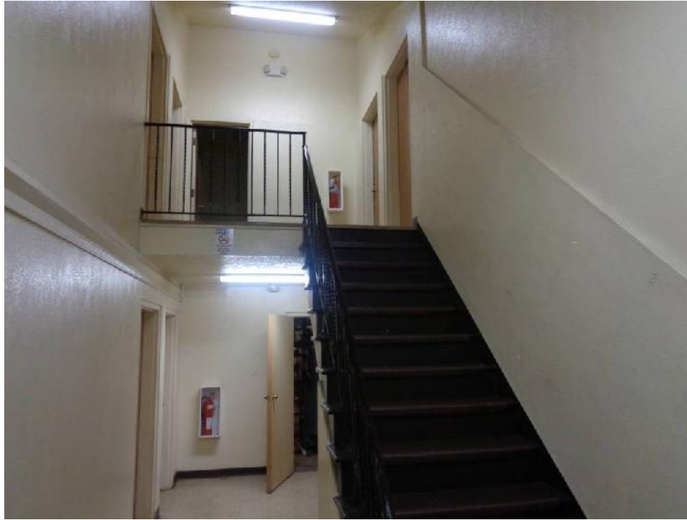
Photo 5: View of common area hallway showing first floor beige floor tile (FTA, non-asbestos) and drywall (DWB, non-asbestos) of 345 Oak View Court.
