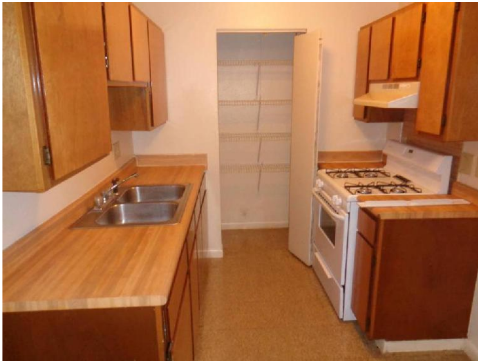
Photo 24: View of beige floor tile (FTB, mastic is asbestos containing) from the kitchen of Unit C of 9842 Oak Place Court.
