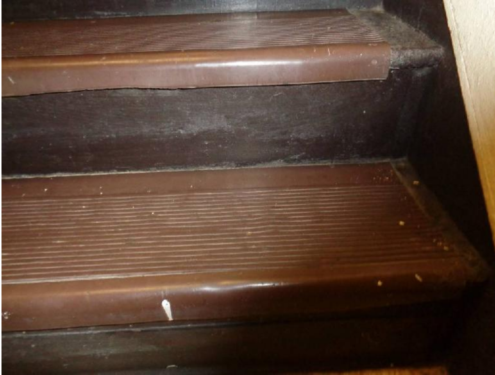
Photo 9: Typical view of brown stair tread (STA, non-asbestos) found throughout facility common areas.
