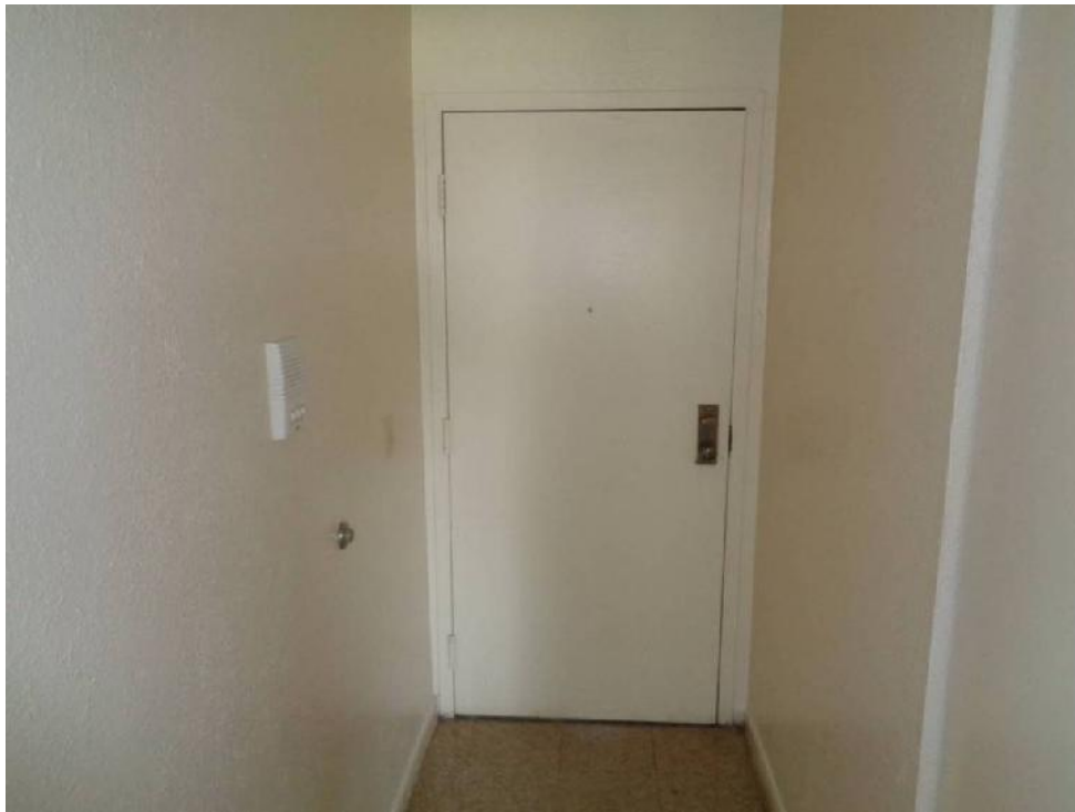
Photo 22: View of entry door and drywall (DWA, non-asbestos) from Unit C of 9842 Oak Place Court.
