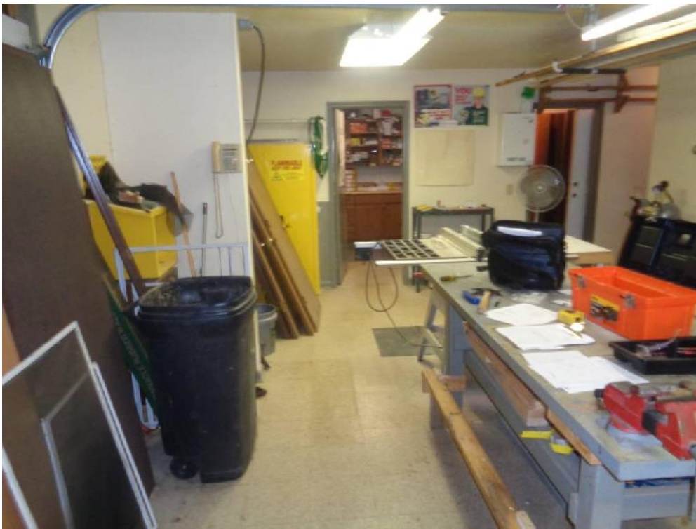
Photo 16: View of beige floor tile (FTA, mastic is asbestos containing) found throughout the Oak View Court maintenance building.
