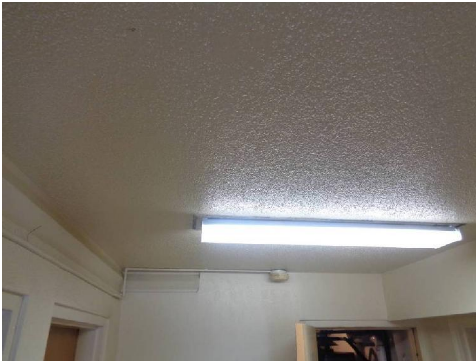
Photo 6: View of ceiling texture (CTA, non-asbestos) in common area hallways in 345 Oak View Court.
