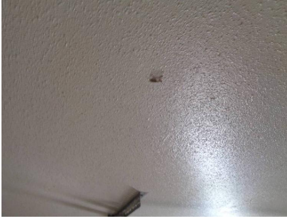
Photo 17: View of white ceiling texture (CTA, asbestos containing) found throughout the Oak View Court maintenance building.
