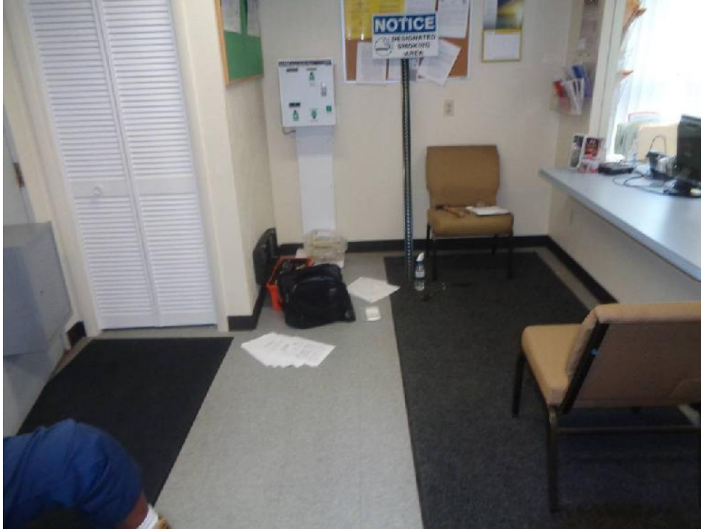
Photo 11: View of gray floor tile (FTA, mastic is asbestos containing), brown cove base (CBA, non-asbestos), and drywall (DWA, non-asbestos) in the entryway of the office building.
