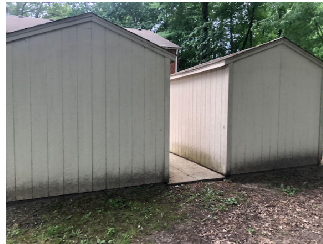
TYPICAL BACK AND SIDE OF DETACHED STORAGE UNITS. REMOVE MILDEW ON SIDING PRIOR TO PAINT
