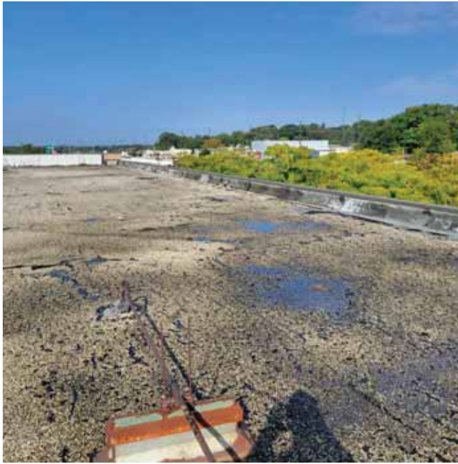
Photo 11: View of the West portion of the roof, note the standing water
