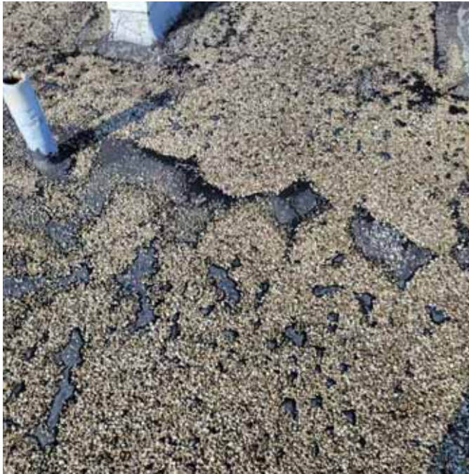
Photo 13: View of bubbling of the roof field
