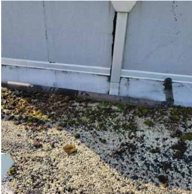
Photo 20: View of moss growth on the North side of the elevator penthouse
