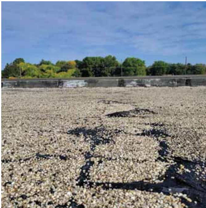
Photo 18: View of pinching/bubbling of the roof field
