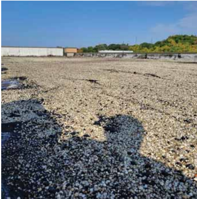
Photo 17: View of pinching/bubbling of the roof field
