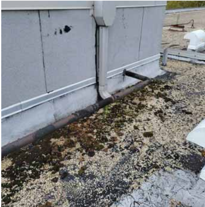
Photo 26: View of moss growth on the North side of the elevator penthouse
