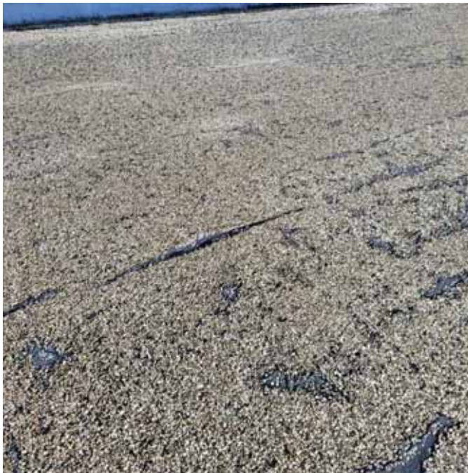
Photo 14: View of pinching/bubbling of the roof field
