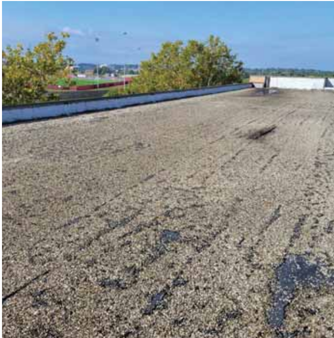
Photo 15: View of pinching/bubbling of the roof field
