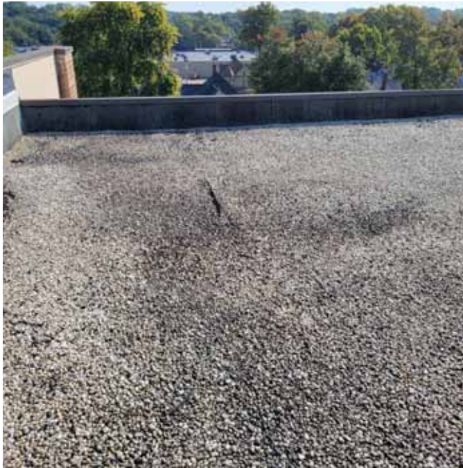
Photo 12: View of the roof coatings pinching/raising
