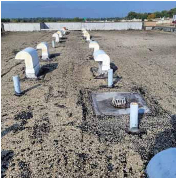
Photo 16: View of pinching/bubbling of the roof field
