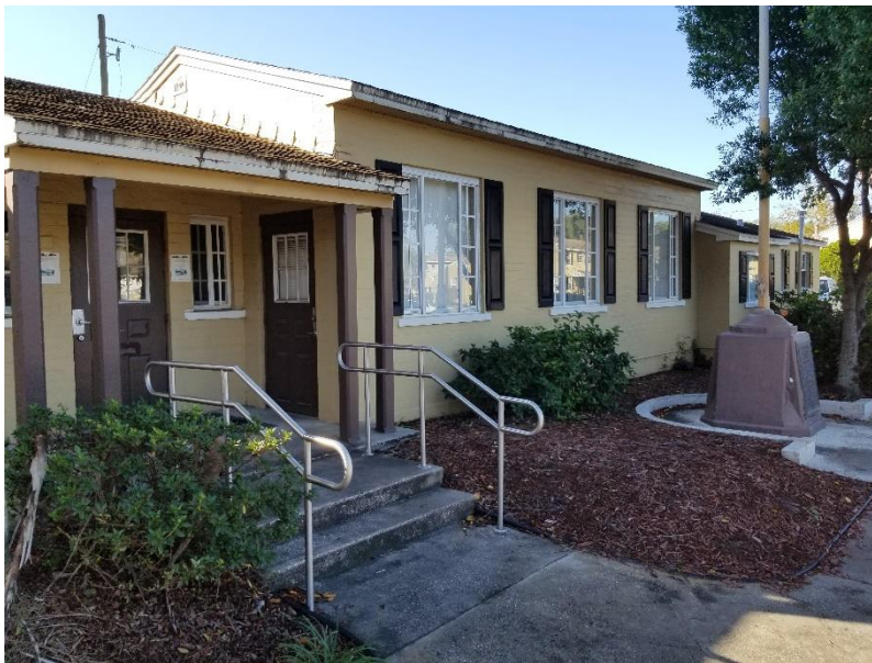
XRF-6 Exterior Office Building Side A Column Brown Paint on Stucco (LCP)
