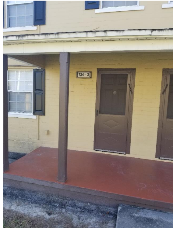
XRF-330 –Exterior Building 724-2 Brown paint on Stucco (LCP)
