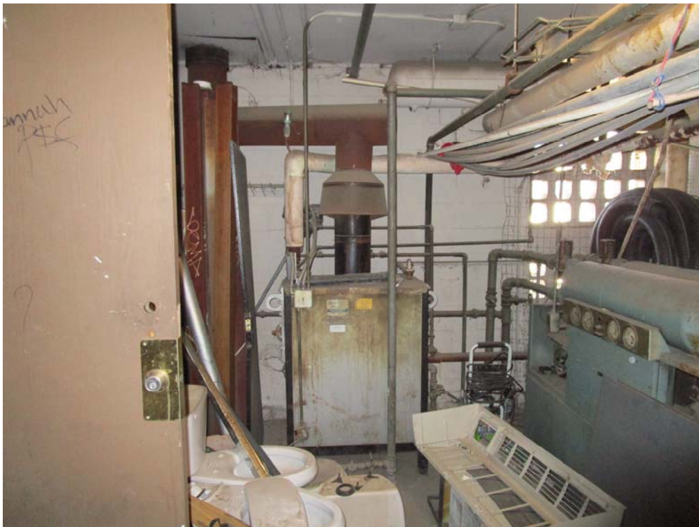
Photo 10: Boiler room on first floor in central portion of subject site.
