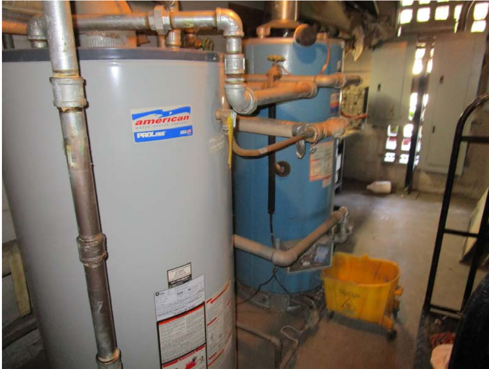
Photo 11: Boiler room on first floor in central portion of subject site.
