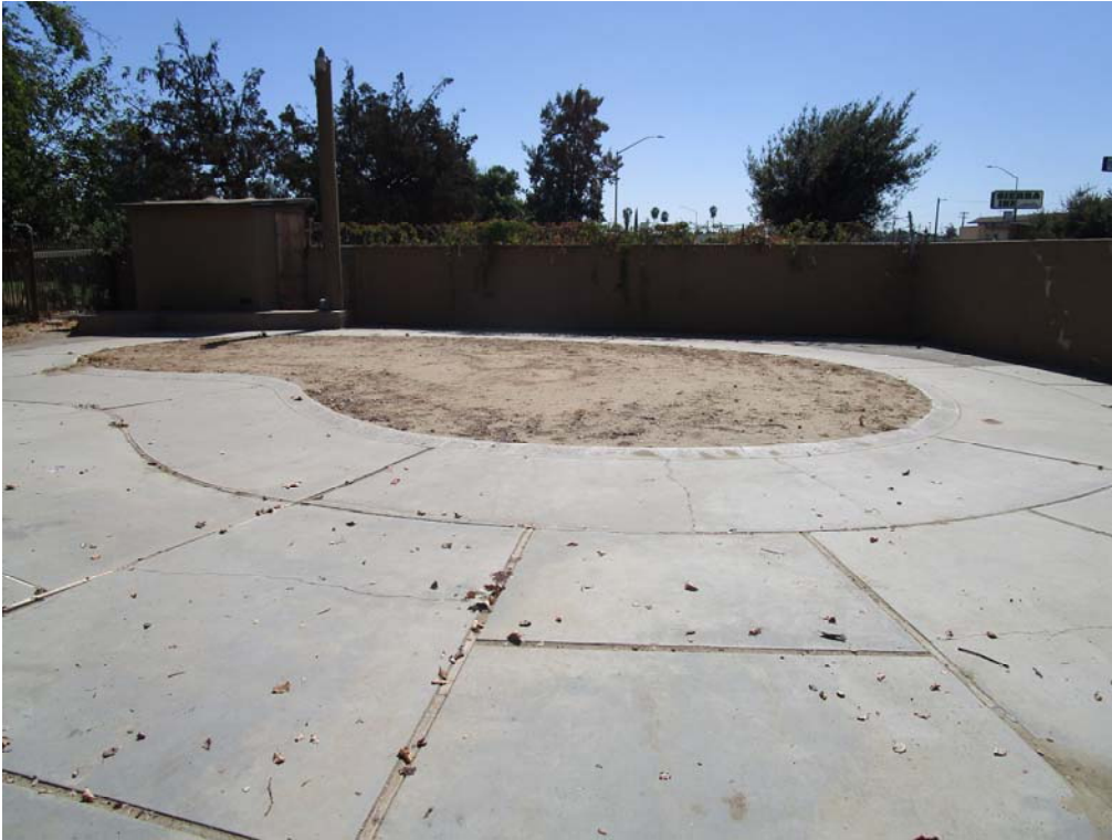
Photo 17: Southern portion of subject site. In-ground swimming pool filled with soil in foreground. Boarded-up equipment shed in background.
