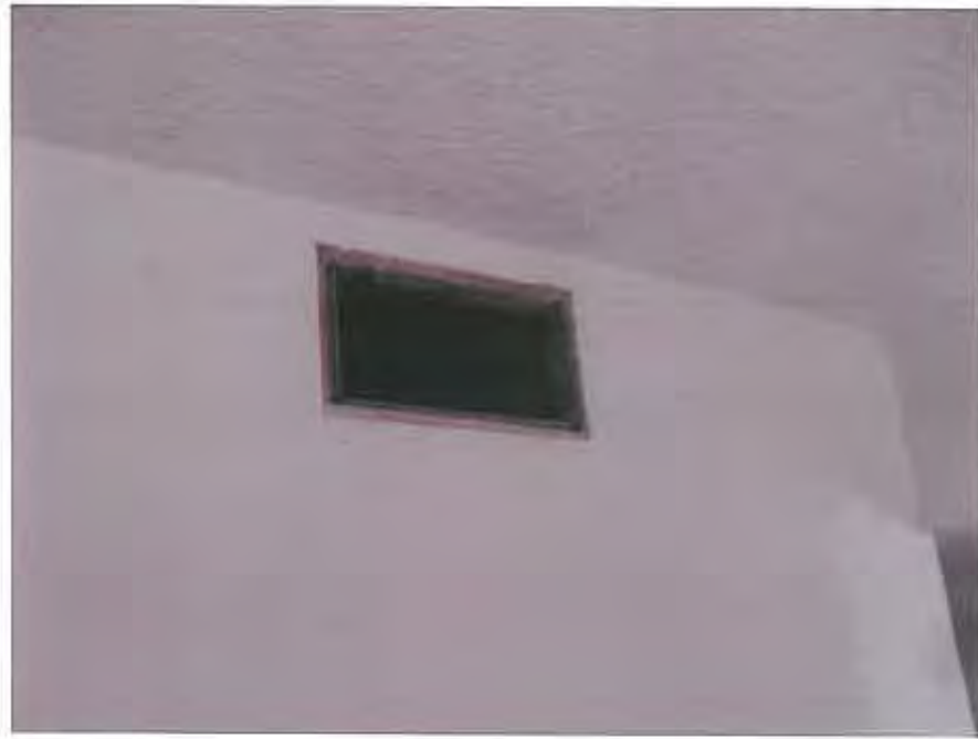
Picture 3: View of acoustic ceiling (ACM) and drywall and joint compound walls (ACCM). In the interior of the units.
