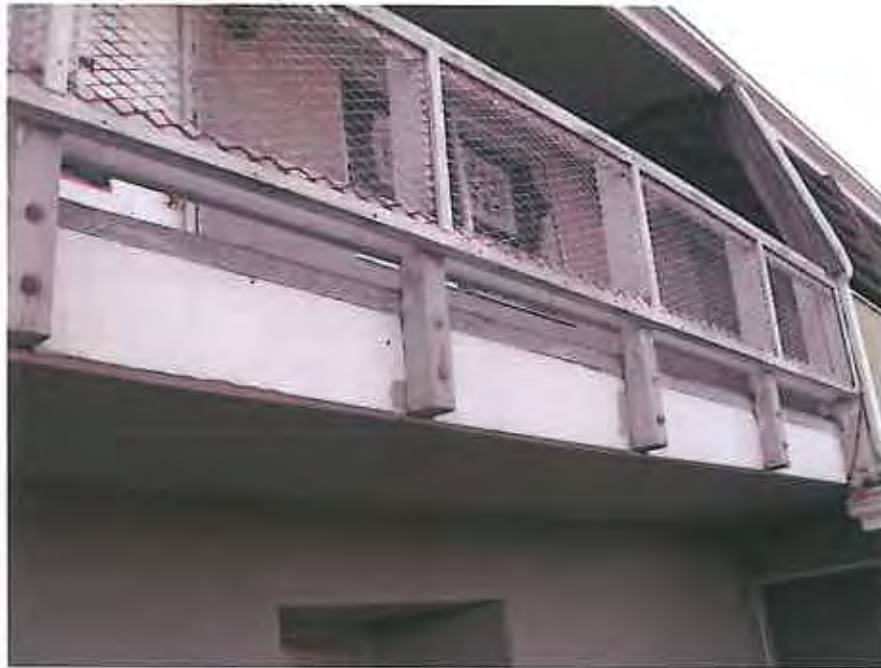
Picture 6: Wood Hand Rail Frame and Posts at 2 nd Floor, Courtyard side. Note damaged LBP and Wood Wall Top (Hand) Rail under louvers.
