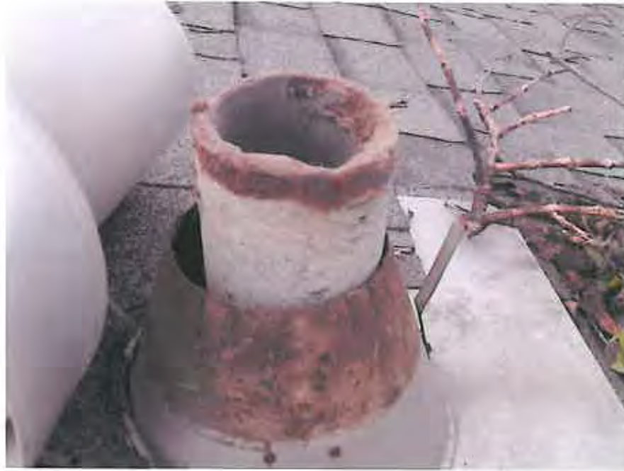
Picture 1: View of 1 of 12 transite pipes as seen from the roof of the Property buildings (ACM).
