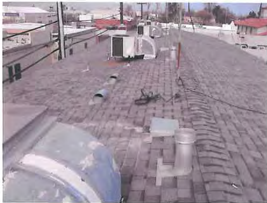
Picture 2: View of HVAC mastic and roof penetration mastic (patches) as seen on the roof of the Property buildings (ACM).
